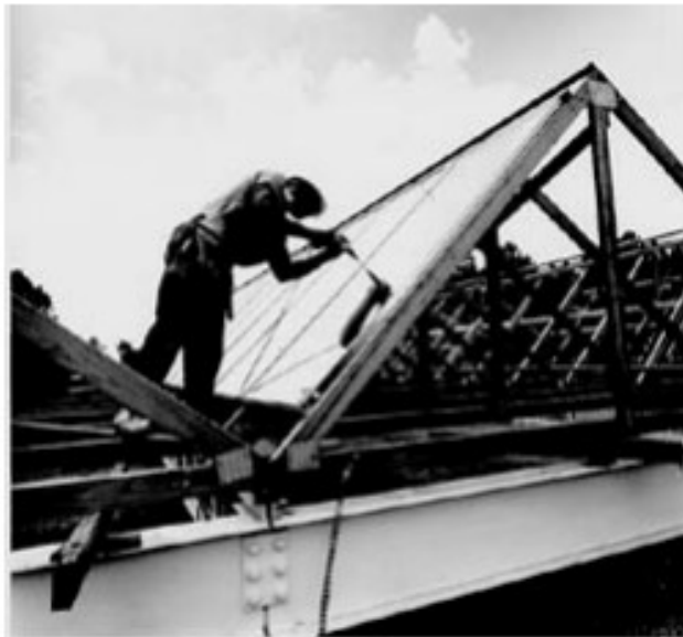
Dedication of the nation's largest solar heating and cooling system, currently in operation, took place November 26, 1975, at the George A. Towns Elementary School in Atlanta, Georgia. Solar collector panels mounted on the roof are pictured during construction.
