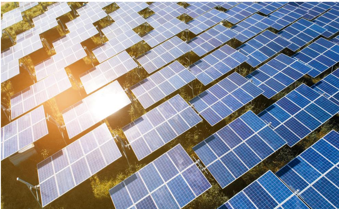
Figure 2 An example of Photovoltaic Panels
